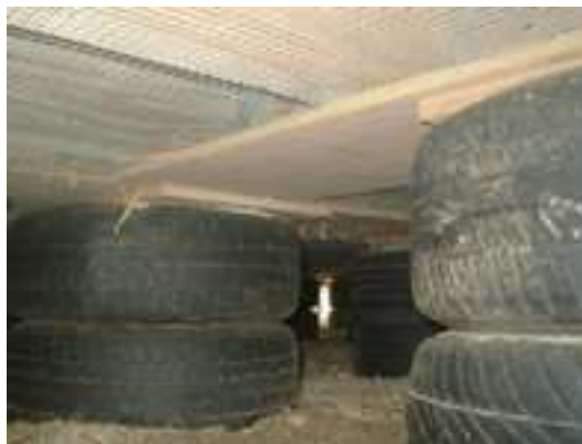
Figure 3: The elevated ground floor insulated with straw bales rests on foundations from recycled tires. Those are filled with rammed gravel. Picture of Straw Bale Dormitory in Clow Back (Yorkshire) build by Amazon Nails in 2002. Photography by Konrad (Tugby, 2002)
