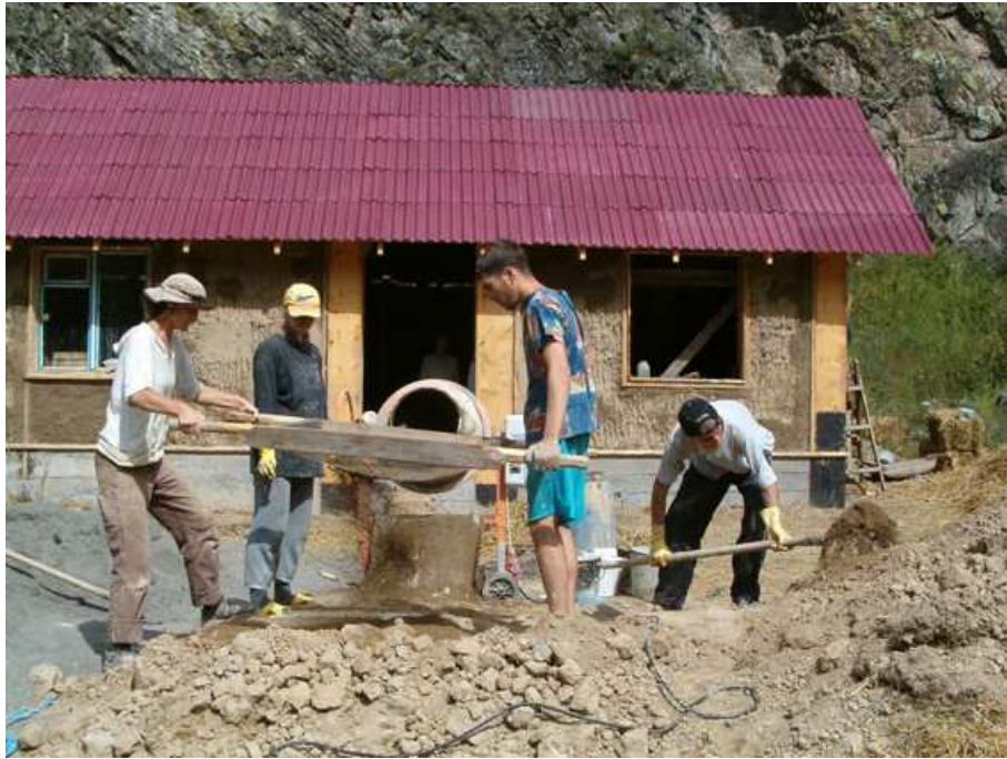
Figure 13: After I left, "Cindy coordinated all of the volunteer labor to apply large quantities of cob and earth plaster to the walls, while Paul and Jeff put the recycled, corrugated, plastic roofing up." Jeff Ruppert (photo by Fund for 21st Century Altai)
