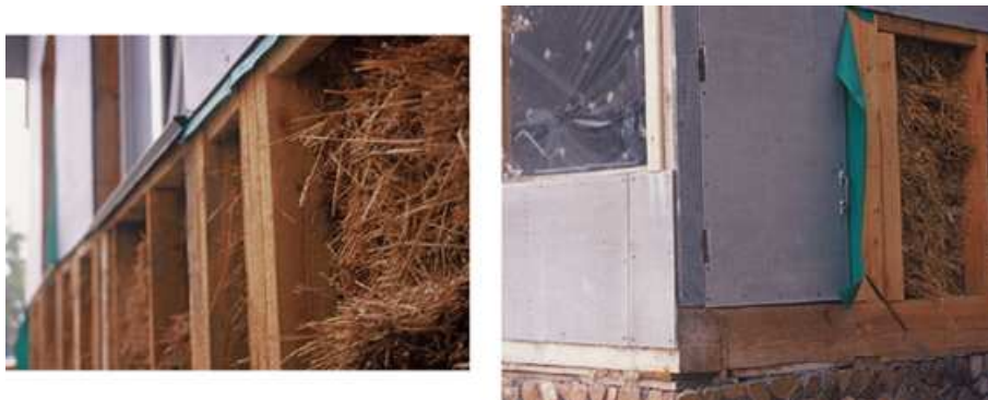
Figure 1.2: Poorly compacted straw bales behind the asbestos sheeting. Note the green wind barrier behind the sheeting and 50mm gap between the asbestos and bales.
