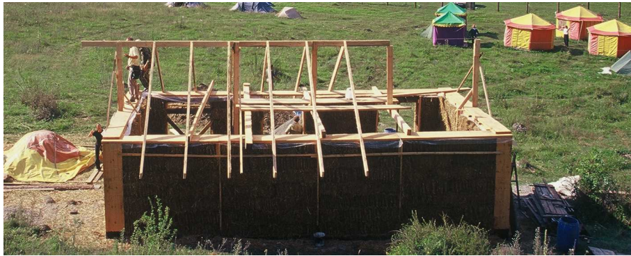
Figure 4.3: The roof plate is a straight massive timber board laid flat on top of the walls. Note the plastic between the plate and the top of the straw bale walls.
