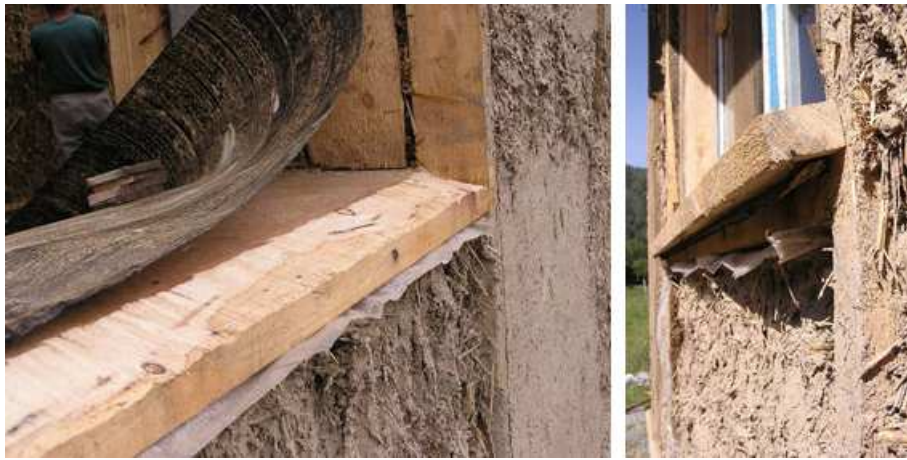
Figure 11: Window sill detail requires special care. Here it was covered in plastic and bitumen sheet prior to placement of wooden board. Note the drip edge on the right photograph - it was carved at the bottom of the window sill board. (photo by Jeff Ruppert)
