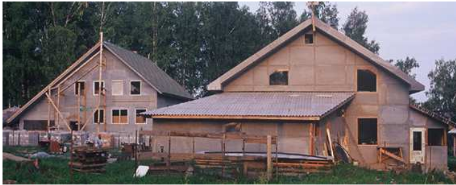
Figure 1.3: Vladimir's straw bale house on the right. The garage creates buffer space and protects the house from western winds. Igor's house is on the left.
