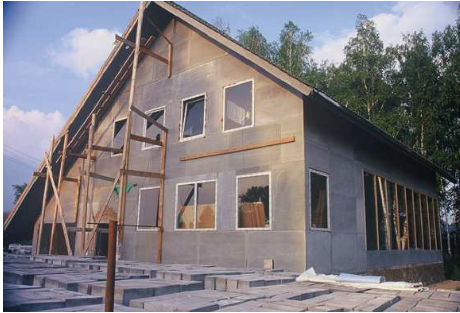
Figure 1.1: Igor's straw bale house in Ecovillage and the cellular concrete blocks stacked in front of it. Note the garage protecting the north side of the house and the south facade with a solar air collector. Warmed air (by solar passive gain) should circulate around the superinsulated envelope of the house, in order to lower the exterior air temperature (there is a crawl space under the ground floor and the cavity between roofing from recycled plastic tiles and the roof insulation). This way, the house envelope faces continuous buffer space instead of exterior air. However, the design proved to be ineffective, due to very cold weather and lack of sunshine in the winter. The air collector is going to be used in a different way - as a trombe wall.
